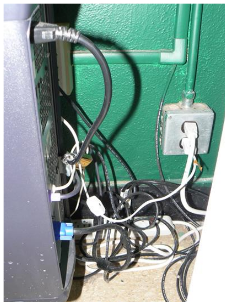
Overloaded electrical outlet
