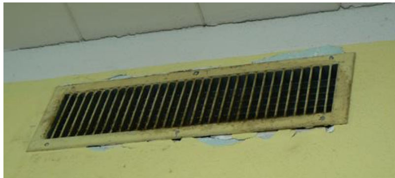
Vent with chipped paint.
